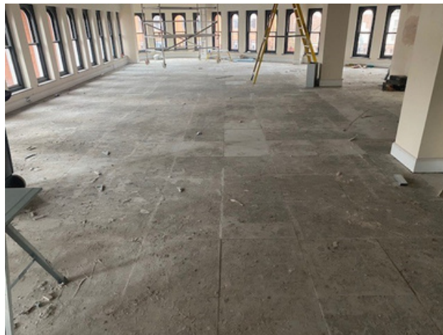
Contaminated raised metal access flooring after uplifting flooring installed using adhesive
