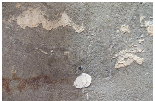
Adhesive contamination of concrete sub-floors
